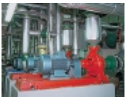
Pumping and ventilation machines
