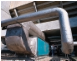
Pumping and ventilation machines
